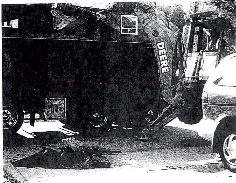
Photo 1 – Traditional utility service cut.
